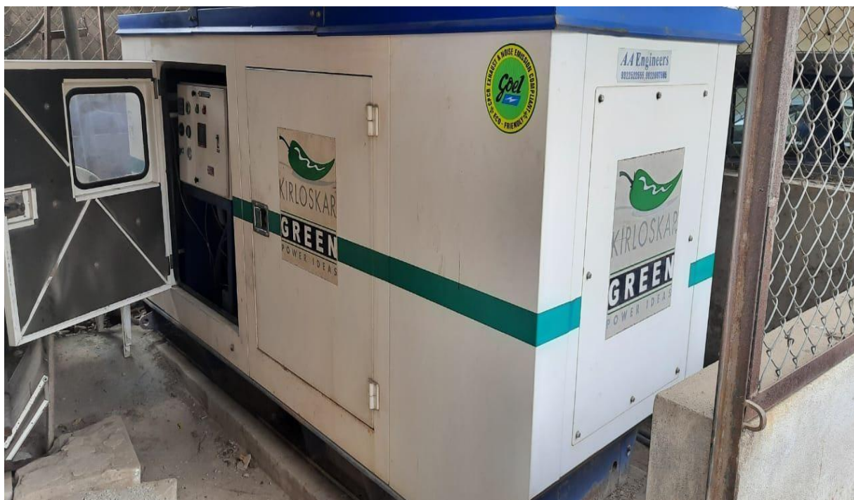
Plate No. 10: Green Power Generator operated on Diesel at college campus.
