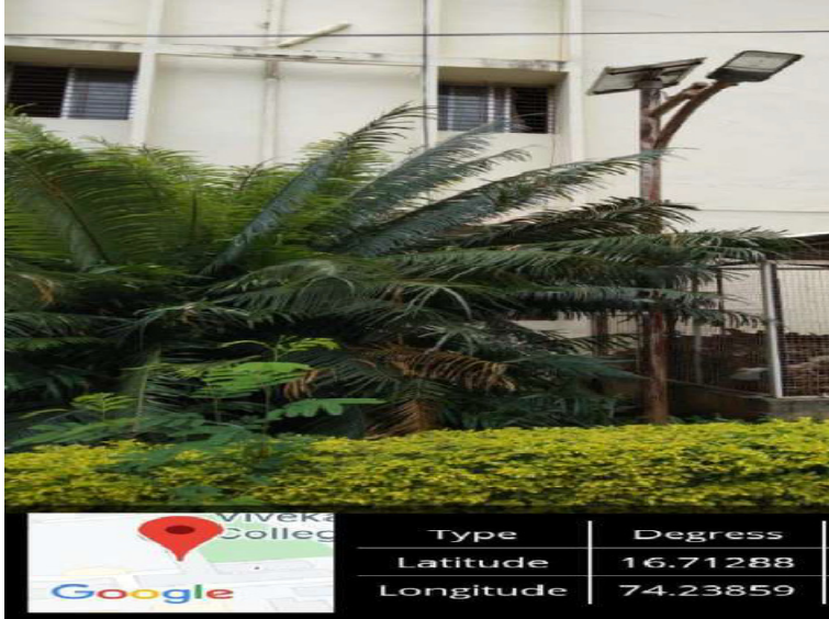
Plate No. 04 Solar Photovoltaic street lamps at Campus
