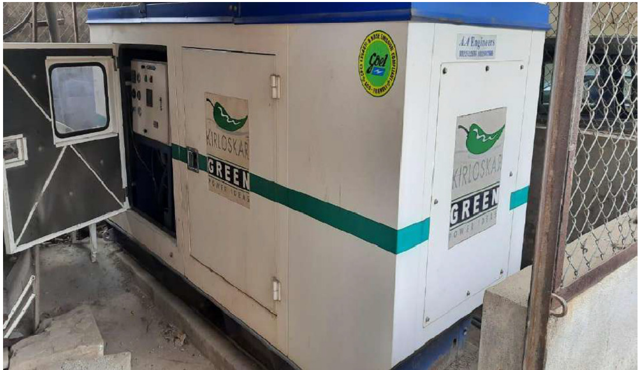
Plate No.2: Generator operated on Diesel at college campus.
