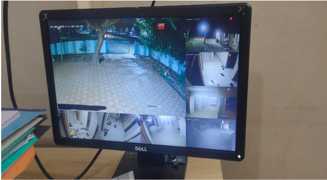
CCTV- Panel for Security
